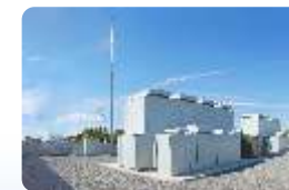
储能 Energy storage
